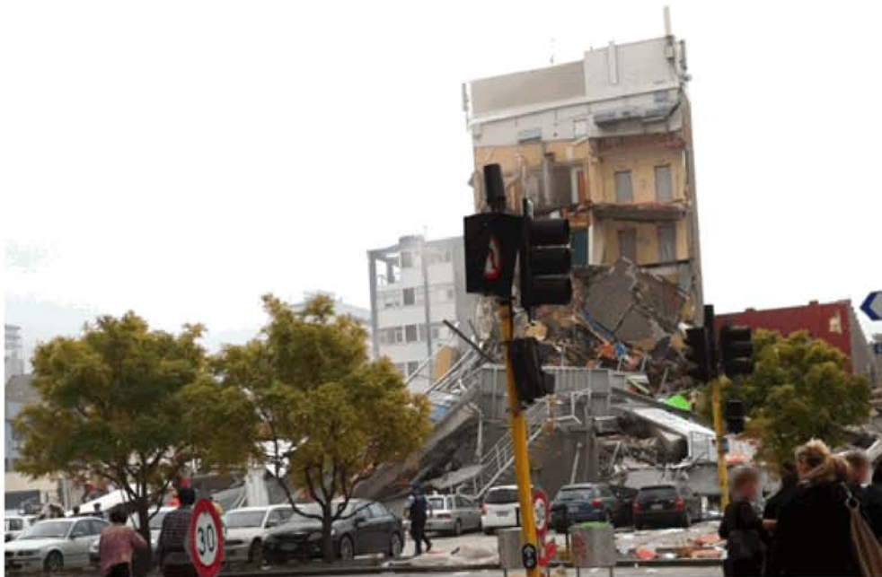
Figure 31 - Cashel St. south face with North Core tower in background immediately after collapse and prior to the fire starting. The cars in the car park on the south face were largely undamaged. The white escape stair that was attached to the South Wall can be seen still attached to the wall as it lay on top of the collapse debris.
