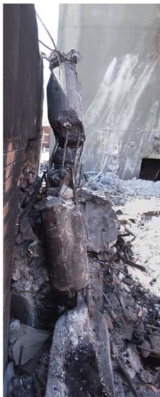
Figure 40 - Line 4 / B column with precast log beam in foreground and shell beam at rear. The column may have broken its back on a precast concrete Spandrel Panel and sustained head damage during the collapse.
