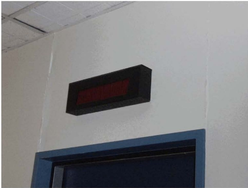
Figure 25 - Damage to wall Linings after 4 September 2010 Earthquake.
