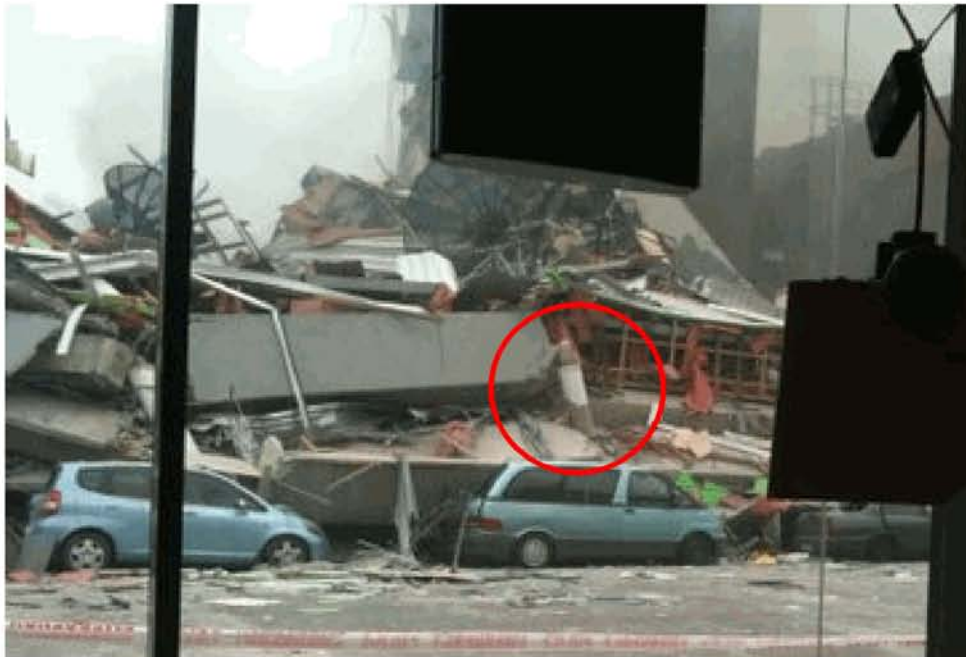
Figure 33 – View looking west across Madras Street. A Line F/3 column is highlighted showing conical fracture in the painted portion, above unpainted portion which had been enclosed by Spandrel Panels.
