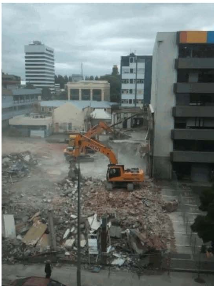
Figure 29 - Heavy machinery demolishing the building adjacent to the CTV Building after the 4 September Earthquake. The boundary wall is still in place covering the Line A infill masonry wall of the CTV Building.
