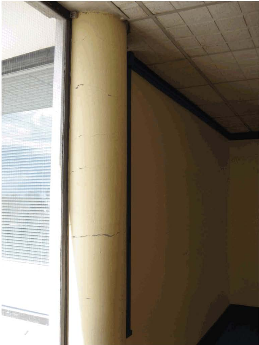
Figure 22 - Level 6 400mm diameter columns Column 4 D/E outside lift with horizontal cracking.
