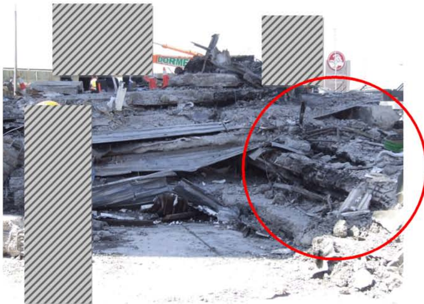
Figure 39 - Line 2 beams highlighted laying rotated northwards. This appears to indicate that the Line 2 columns collapsed prior to the slabs breaking away from the Line 1 South Wall and frame.
