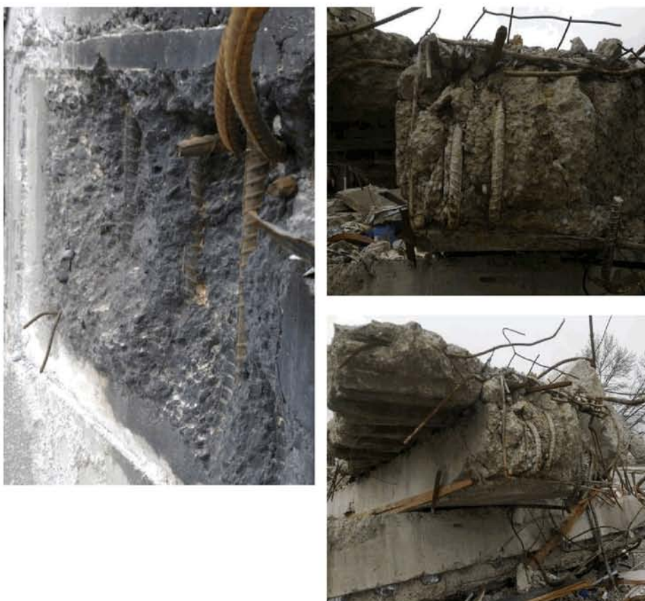
Figure 44 - Precast shell beam (Item E14) from northern face Grid 4, west side of North Core (DENG B23 Dwg S18). (clockwise from top right) (a) to (b) Fractured slab outstand remnant at east end from which slab concrete cores were extracted. The bottom H24 bars from shell beam have been turned back into the concrete infill rather than embedded in shear wall as detailed (DENG Detail 5 Dwg S19). Notice the bar imprint on wall at the connection seen in (c) at Level 4 and at Level 3.
