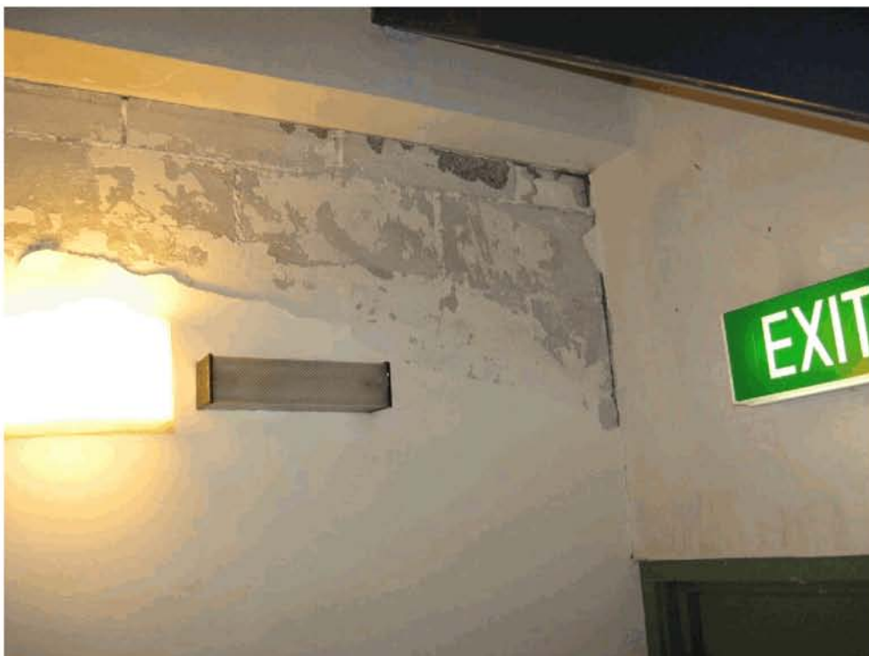
Figure 24 - (Top to bottom) (a) Fine cracking in floor at junction with South Wall; (b) Spalling of plaster finishes on internal masonry in-fill wall on Line 4 in front of stair well.
