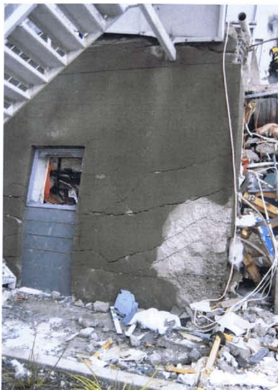
Figure 41 – Angled fan-like flexural cracking on the South Wall in conjunction with spalling on the outside face at the east end. This indicates that the South Wall may have suffered flexural / compressive damage prior to the collapse.
