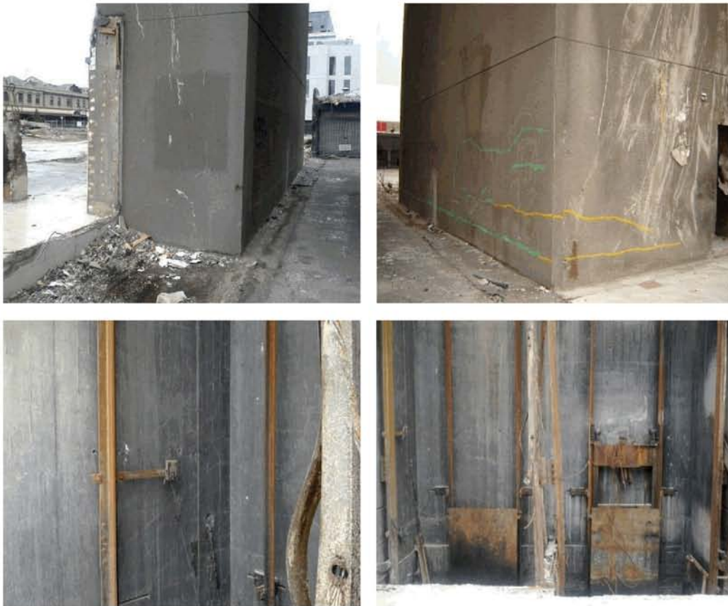
Figure 42 - North Core cracking (clockwise from top left) (a) No obvious cracking on Line D/E wall; (b) Horizontal flexural cracking on west and north west face of Line 5 wall and north end of Line C wall at Line C/5; (c) Fine two-way diagonal cracking on the inside faces of Level 1 to 2 Line 5; (d) and D walls in North Core.
