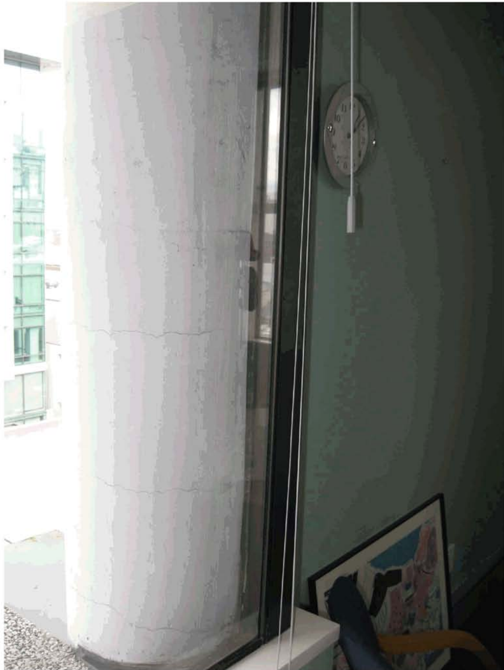
Figure 23 - Level 6 400mm diameter Column on Line I/A-B with horizontal cracking.
