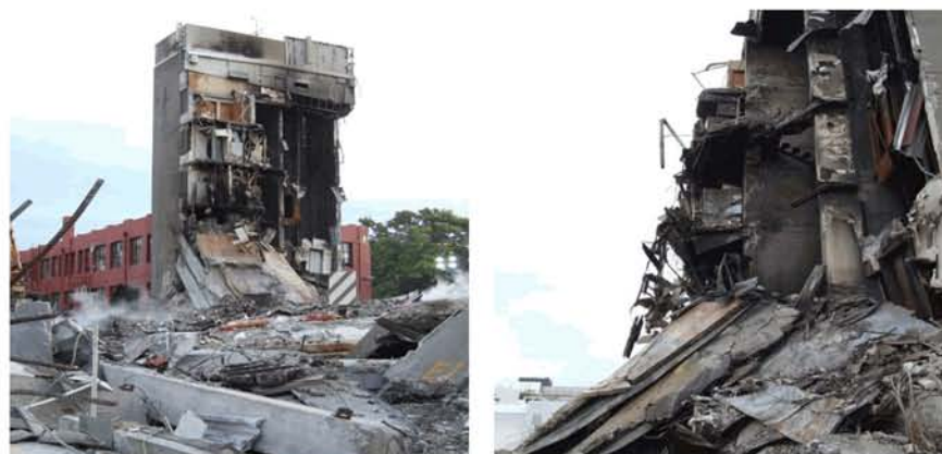
Figure 38 – View of North Core showing Level 4 slab lying diagonally on top of Level 3 slab. This indicates that the Level 3 and 4 slabs lost their vertical support on Line 3 prior to breaking away from the North Core.
