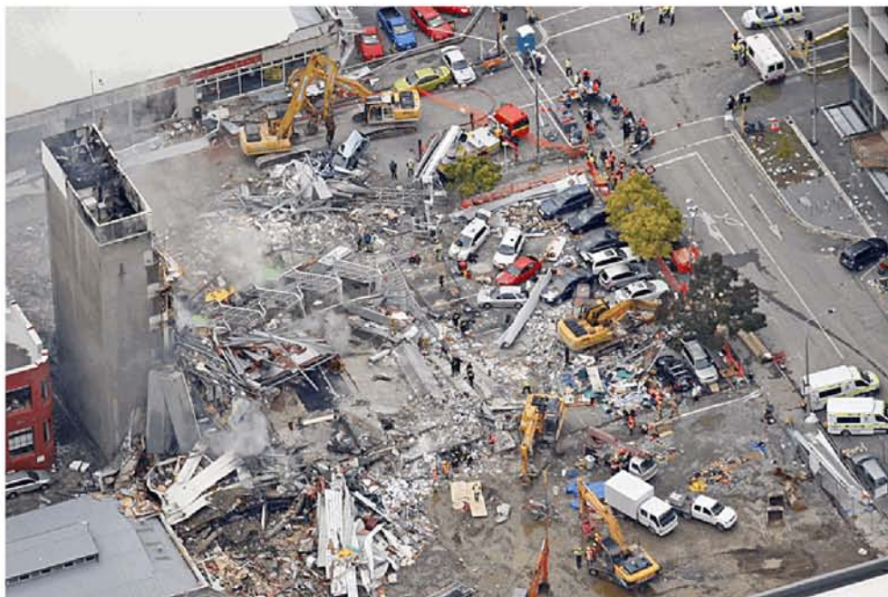
Figure 6 - The CTV Building collapse shortly after machinery began to remove debris. ( NZ Herald)
