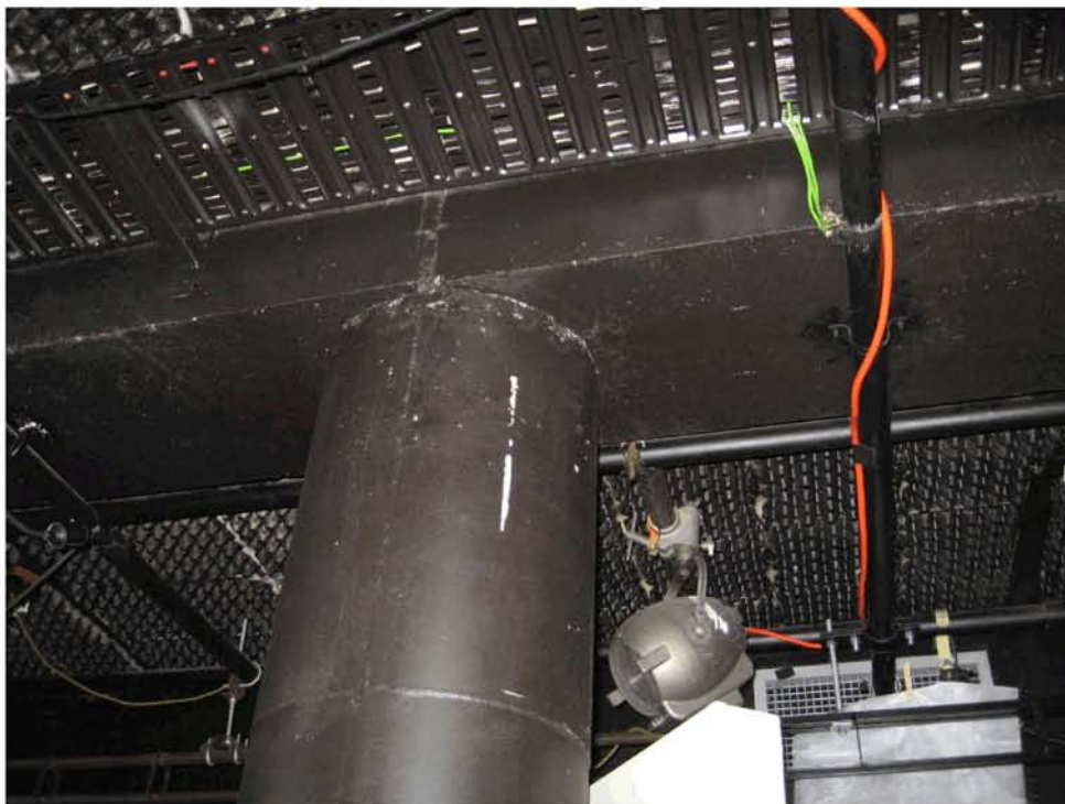
Figure 26 – Internal 400mm diameter column and beam after 4 September 2010 Earthquake. No visible cracking evident. A horizontal circumferential formwork mark can be seen approximately 600 mm down from the underside of the beam indicates it was a Level 1 column which were constructed using extensions to the formwork shutters.
