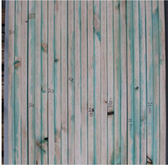
Figure 11 – Copper naphthenate ‘brush on plus injections between the studs’ units with the plaster board removed (showing the edges of studs originally attached to plasterboard), starting with unit IC1 on the left through to unit IC8 on the right. The copper naphthenate has penetrated from the injection holes through to the plasterboard in patches but there was little penetration from the brushed surfaces.
