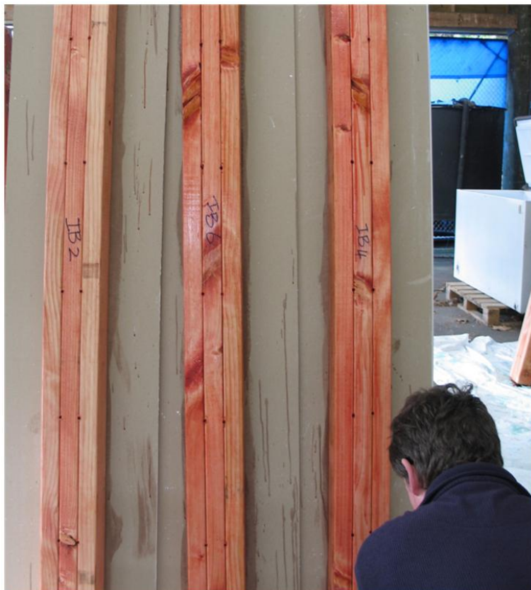
Figure 2 – Brush application of boron to ‘brush on plus injections between the studs’ units. The injection holes are visible between the studs
