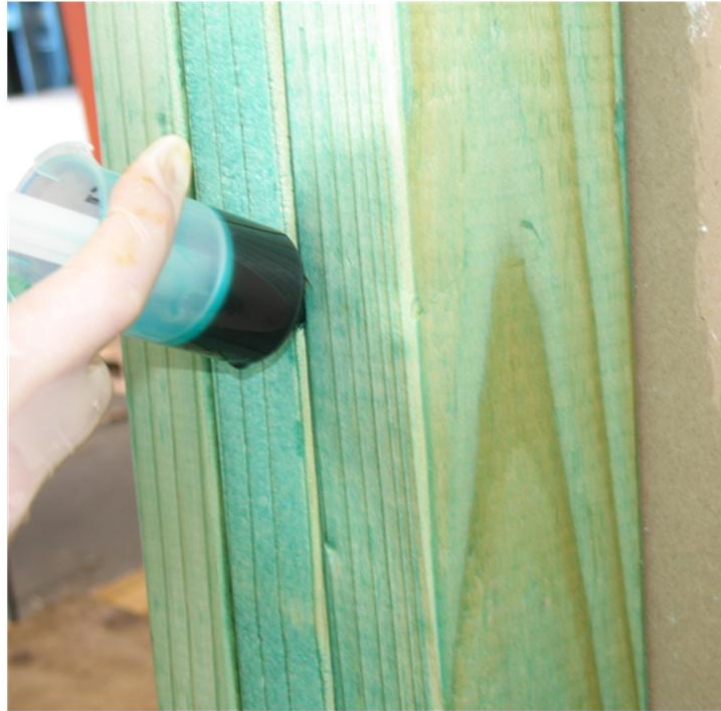
Figure 3 – Injection of copper naphthenate to ‘brush on plus injections between the studs’ units. Injection was done after ‘double coat brush-on’ application using a syringe with a long tapered nozzle.
