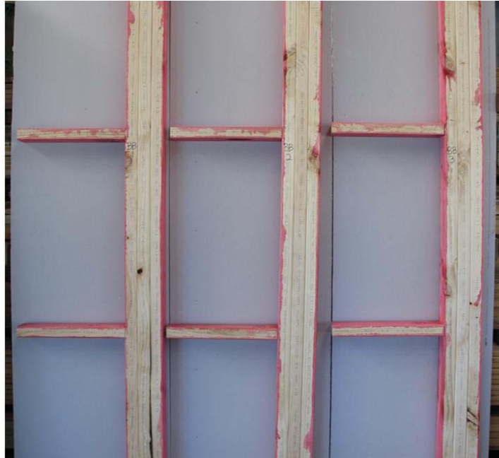
Figure 5 – Boron ‘double coat brush-on’ units with the plaster board removed (showing the edges of studs originally attached to plasterboard) starting with unit BB1 on the left to unit BB3 on the right. Very little preservative had penetrated between the plasterboard and the framing except from the upper face of the nogs. Preservative had not penetrated sufficiently between studs to reach the plasterboard.
