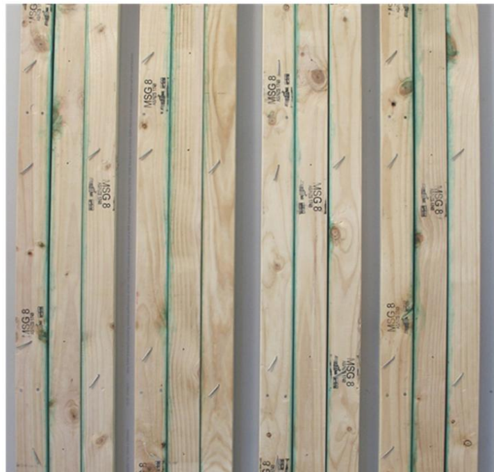
Figure 8 – The concealed faces of ‘double coat brush-on’ copper naphthenate treated studs (after dismantle), unit BC5 on the left through to unit BC8 on the right. Preservative had not spread far from the surfaces that it was brushed on to.
