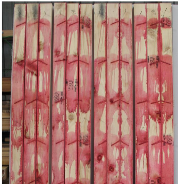
Figure 10 – The concealed faces of ‘brush on plus injections between the studs’ boron treated studs (after dismantle), unit IB1 on the left through to unit IB4 on the right. Preservative had spread out from the injection holes.
