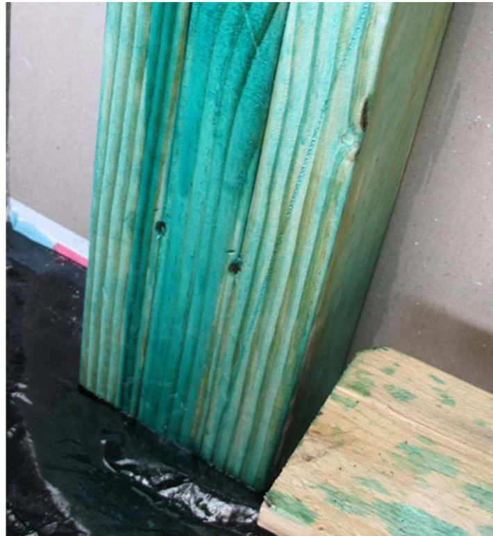
Figure 4 – Injection of copper naphthenate to ‘brush on plus injections between the studs’ units. Preservative tended to run out of the hole and down between the studs to pool on the floor during injection.
