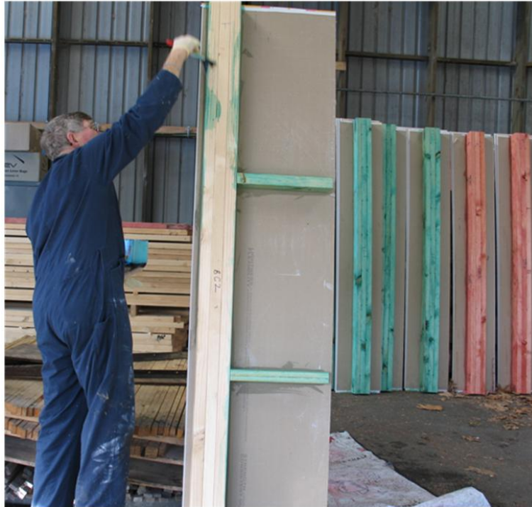
Figure 1 – Brush application of copper naphthenate to brush-on units. ‘Brush on plus injections between the studs’ units stacked for drying are visible to the right background.
