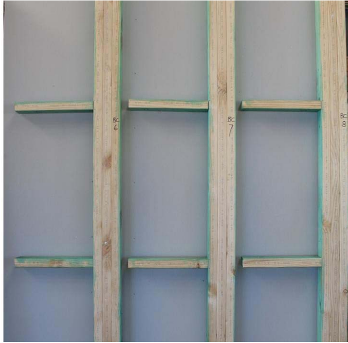
Figure 7 – Copper naphthenate ‘double coat brush-on’ units with the plaster board removed (showing the edges of studs originally attached to plasterboard) starting with unit BC6 on the left through to unit BC8 on the right. Very little preservative had penetrated between the plasterboard and the framing except from the upper face of the nogs. Preservative had not penetrated sufficiently between studs to reach the plasterboard.
