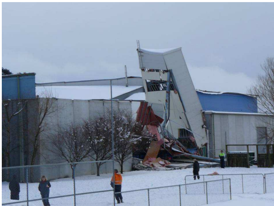
The remains of Stadium Southland's roof in Invercargill (Photo: Malcolm Gayfer, Weatherwatch.co.nz)
