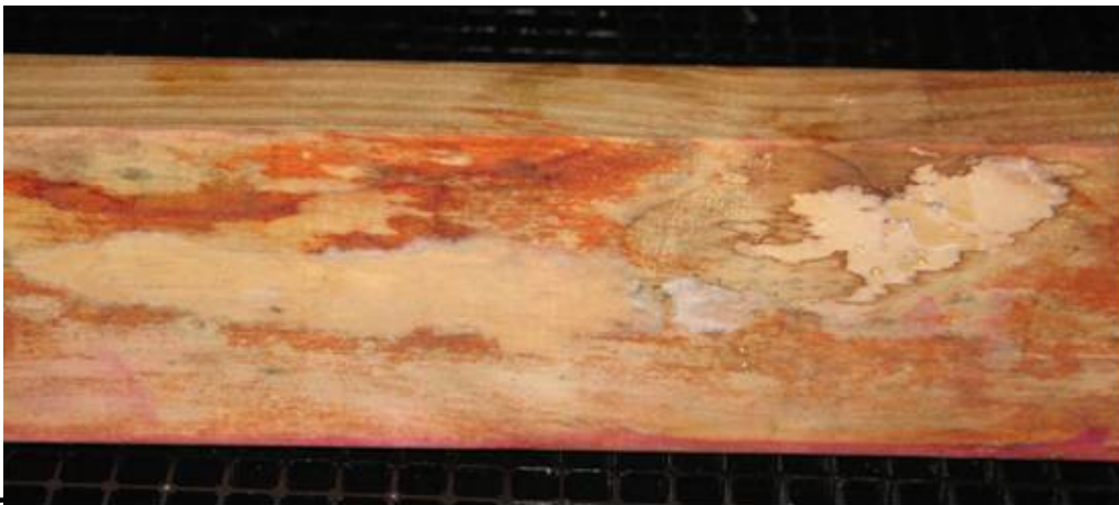
Figure 7 – HMC sample B51H/5, treated with boron on the lower edge, after 10 weeks exposure. Mycelium, decay patches and extensive moulds developing on untreated surfaces around the area of the original infection.
