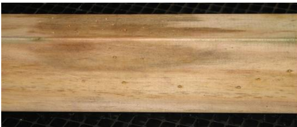
Figure 16 – LMC sample C62L/7, after 52 weeks exposure. Well established decay between the treated edges and deflection had increased by 17%.
