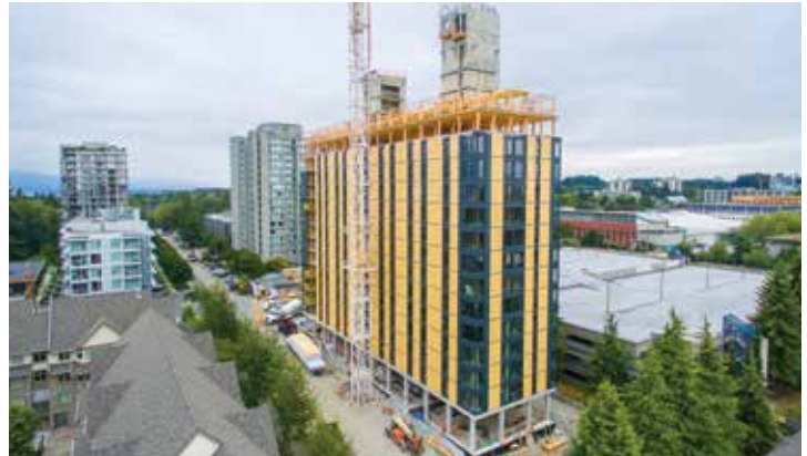
Brock Commons Tallwood House is an 18-storey mass timber hybrid student residence building at the University of British Columbia, scheduled to be completed by Spring 2017.
