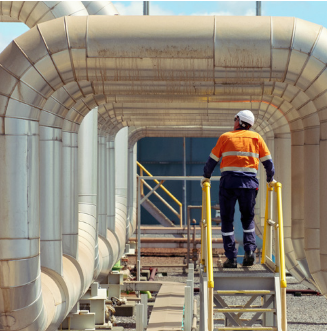
Ngā Awa Pūrua Geothermal Power Station (image supplied by Mercury New Zealand; photo credit: Stephen Wells)
