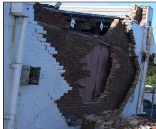
Figure 2.11: Post-13th June 2011 – collapse of inner leaf of cavity wall
