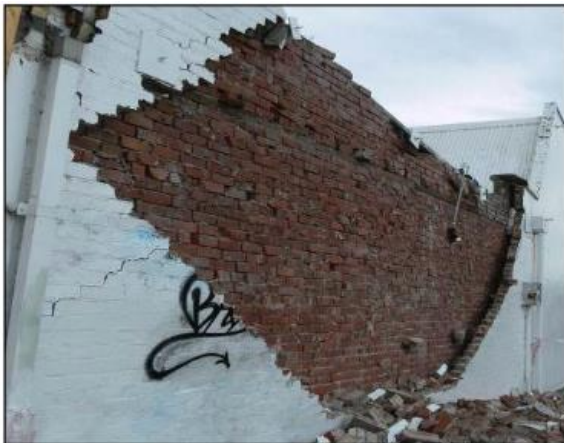
Figure 2.10: Post-22 February 2011 - collapse of outer leaf of cavity wall
