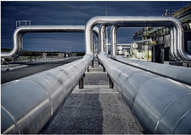
Geothermal Piping Loops, Ngatamariki Geothermal Power Station. Photo credit: Chris Sisarich, NZ Story
