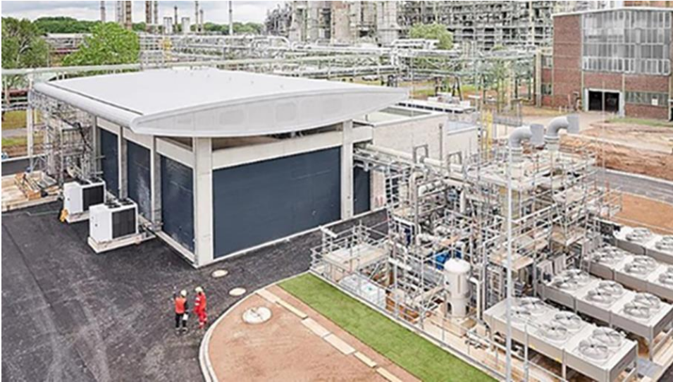
Figure 7-2: 10 MW PEM electrolyser plant example in foreground
