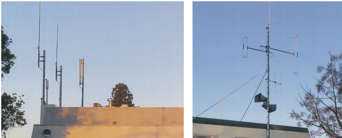
Figure 13: Examples of other non-dish antennas
