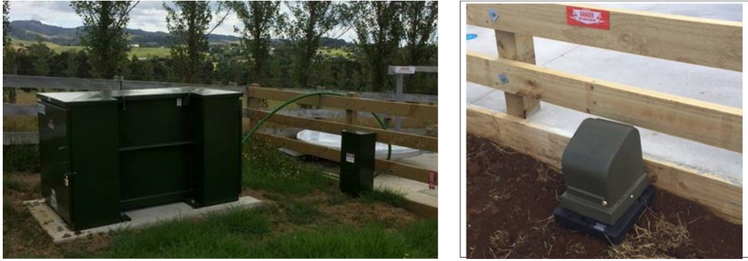
Figure 15: Examples of junction boxes used to supply power connection to cabinets
