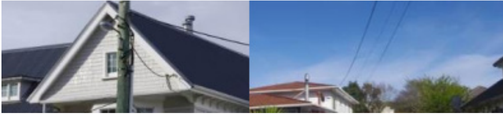
Figure 9: Aerial customer connection lines
