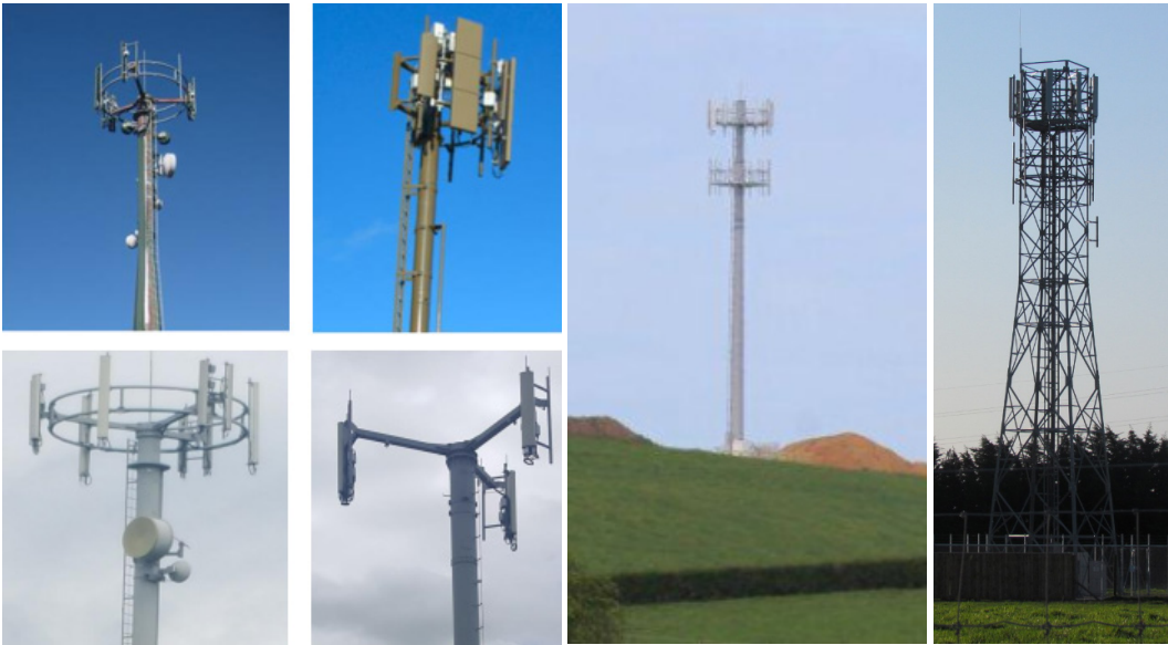
Figure 3: Examples of headframes attached to a pole
