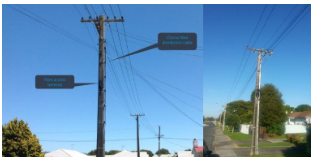
Figure 11: Aerial telecommunication lines
