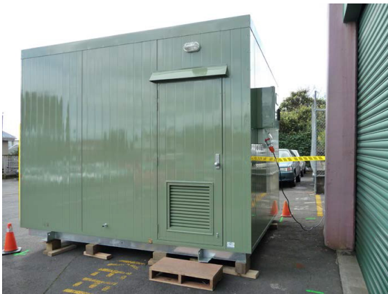
Figure 8: Example of a large telecommunication shelter able to be entered into by technicians
