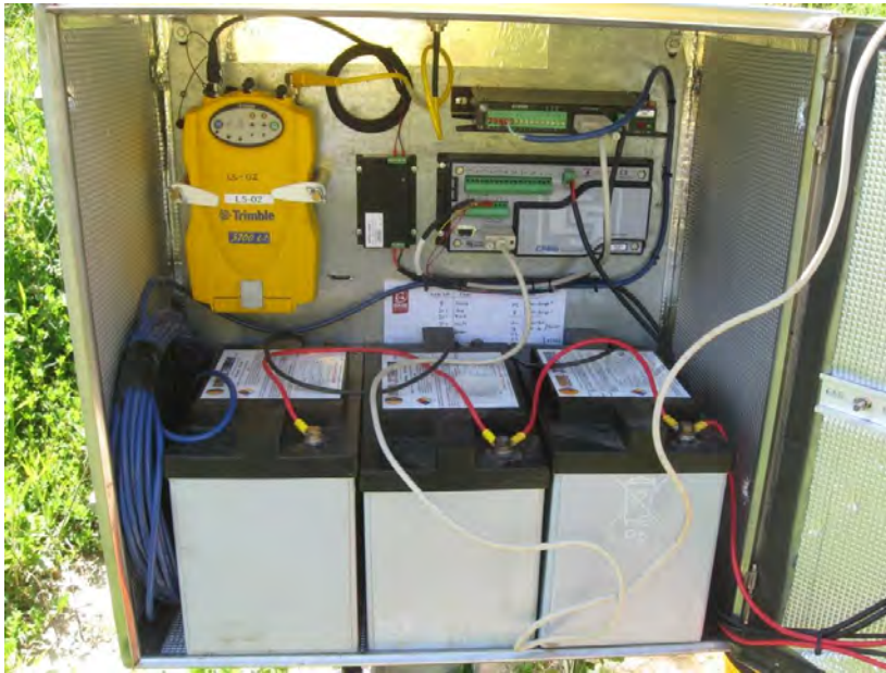
Figure 3: Example of data collection hardware point (source: Vector Gas)
