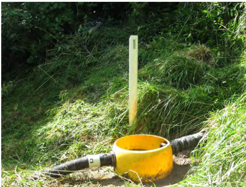
Figure 4: Interception pot for snapshot measuring of drain water flow rate (source: Vector Gas)
